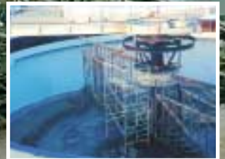
Metal and concrete surfaces of this effluent treatment tank lined with Chemi-Tech EP, a heavy duty corrosion and chemical resistant coating.
